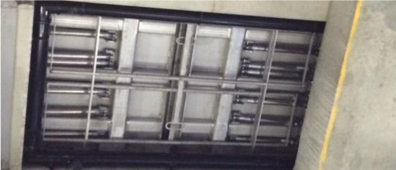
This image shows the underneath of the installed Kent Hinged Multi-Paver in St. Barts Hospital, London.
