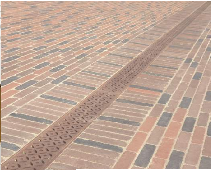
Neat Edge Channel—Canada Water, UK
